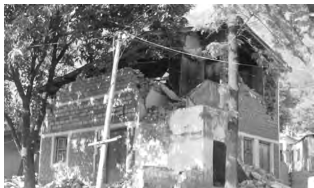
Figure 6.1 : A Damaged Building Due to an Earthquake
